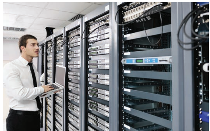
Proper airflow to cool the servers is vital to prevent them from overheating—getting this right depends not only on the heat output of the server, but also on whether the server cabinet is sized properly.
